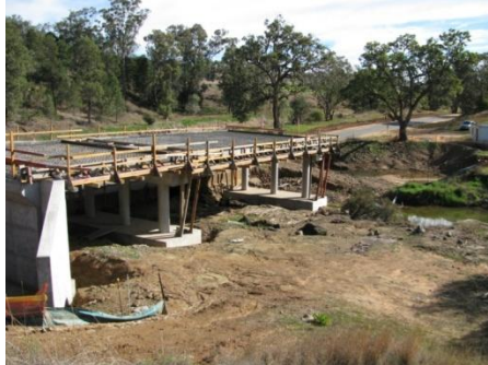
Construction in progress on a new bridge over Saltwater Creek No 2 on Purlewaugh Road
